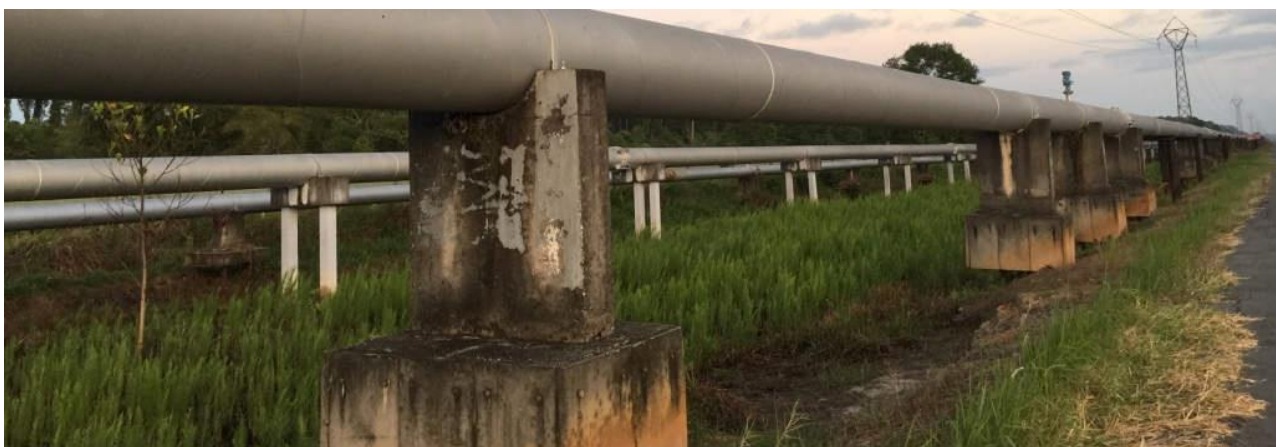
Figure A2. Pilings supporting water pipelines along Jalan Badas. Piles are exposed under pile caps due to peat subsidence.
